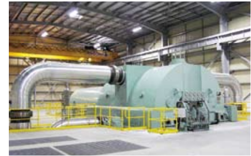
Turbine at Kawerau, NZ (Fuji Electric)
