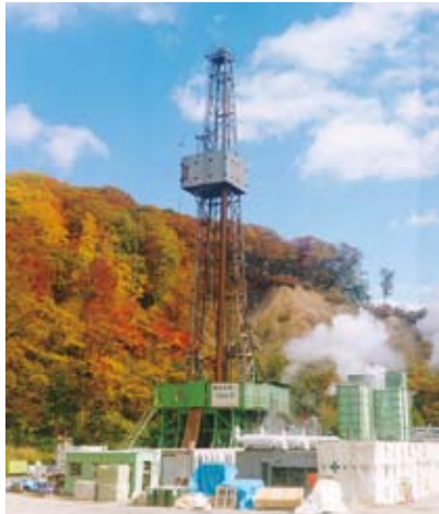
Drilling rig at Kakkonda, which recorded the world highest temperature of 500°C (Geo-E)
