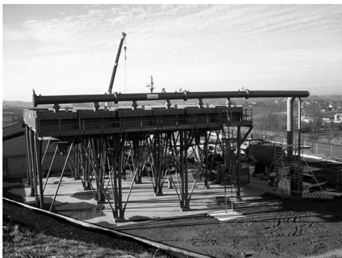
Figure 2. The Soutz ORC power plant: the air-cooling system (on the right) and the turbine (on the left)
