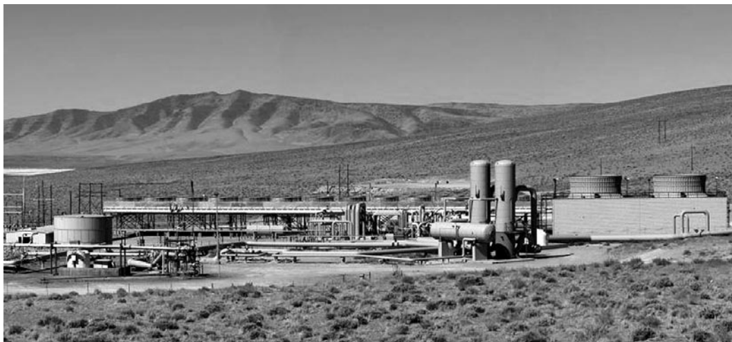
11 MW Desert Peak 2 Geothermal Power Plant at Churchill County, Nevada
