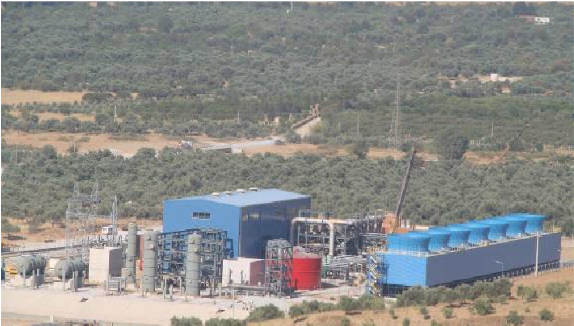
Fig. 2. A general view of Germencik power plant.
