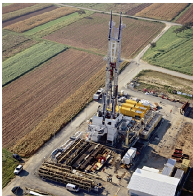
Figure 1: The drilling site of the TI-350 only requires an area of 30 x 80 m.
