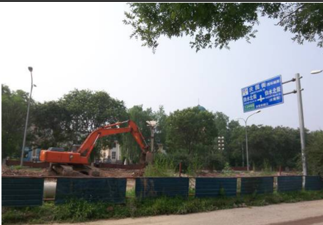
Figure 1: An excavator digging on the main street of a county town in Yanqing County, China
