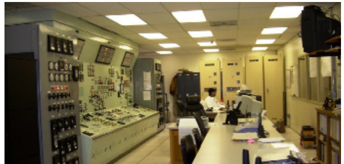
Control room of Calpine's Unit No. 14, named West Ford Flat.
