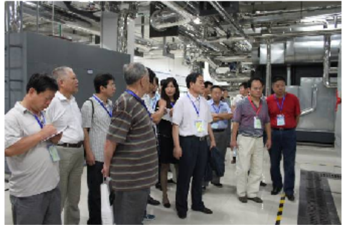
Participants visit the GSHP system in the Urban Gate project
