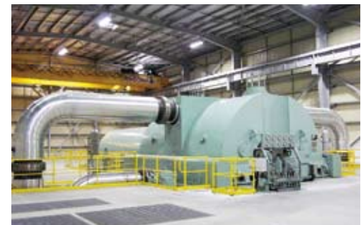
Turbine at Kawerau, NZ (Fuji Electric)
